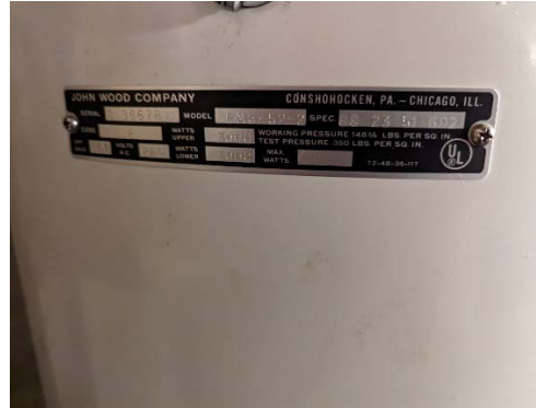
1054 Boston Post Road, Guilford, CT - Interior = Floor Basement – Civil Engineering Storage/Heating and Cooling – Basement – Hot Water Heater
