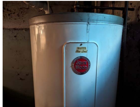
1054 Boston Post Road, Guilford, CT - Interior = Floor Basement – Civil Engineering Storage/Heating and Cooling – Basement – Hot Water Heater
