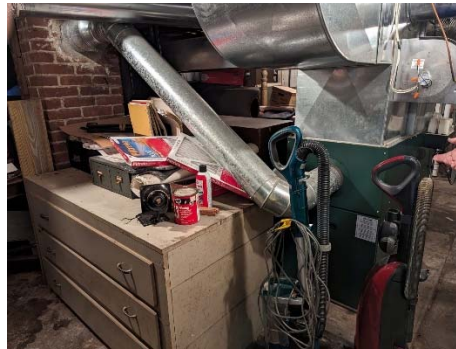
1054 Boston Post Road, Guilford, CT - Interior = Floor Basement – Civil Engineering Storage/Heating and Cooling – Basement – Heating and Cooling
