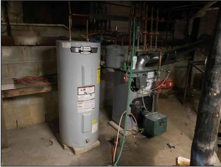
View of Boiler and Hot Water Heater in Basement of the Improvements on Lot 13
