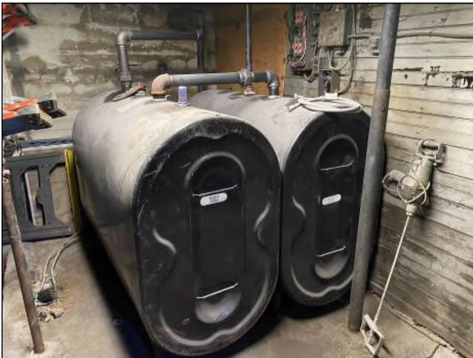
View of Oil Tanks in Basement of the Improvements on Lot 13
