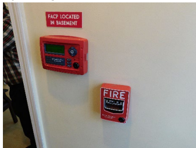
35. Fire Alarm Pull Station
