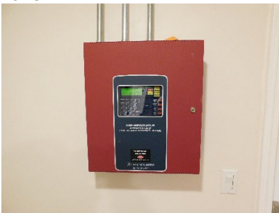
34. Fire Alarm Control Panel
