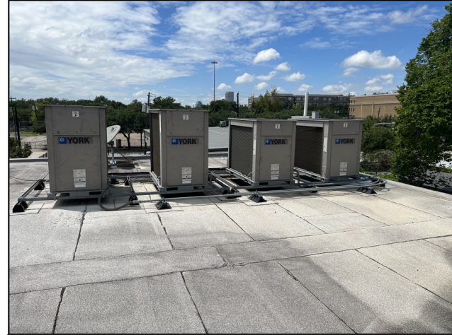
HVAC Units on Roof
