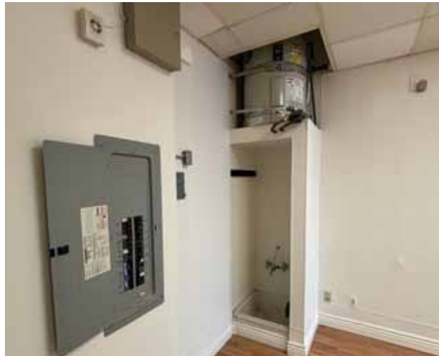
2652-E Interior - Mop Sink & 40-Gallon Hot Water Heater
