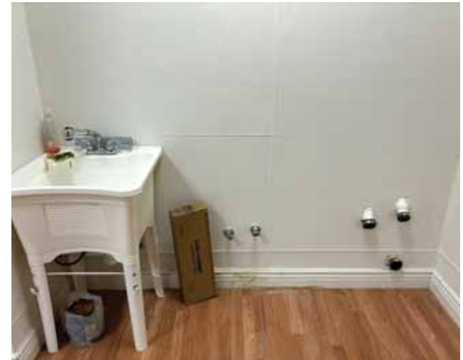
2652-E Interior - Industrial Sink & Plumbing Stub Outs
