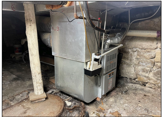
Basement furnace – replaced 3 years ago
