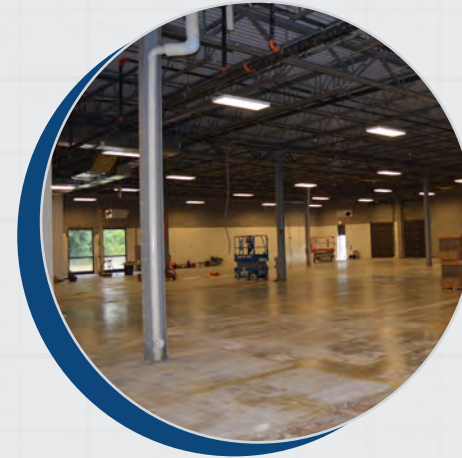
FLEX/WAREHOUSE AREA 16'6" CLEAR HIGH CEILINGS FULLY SPRINKLERED
