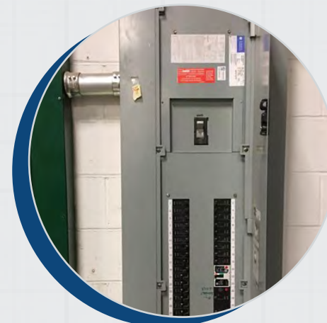
SUFFICIENT POWER 480/277 VOLTS • 1,200 AMPS • 3-PHASE SERVICE
