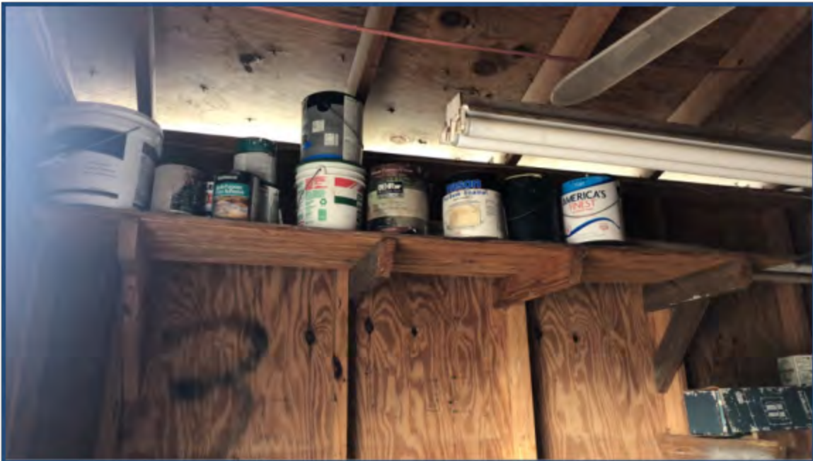
Photograph 32: Interior of Storage Shed containing Paint Cans
