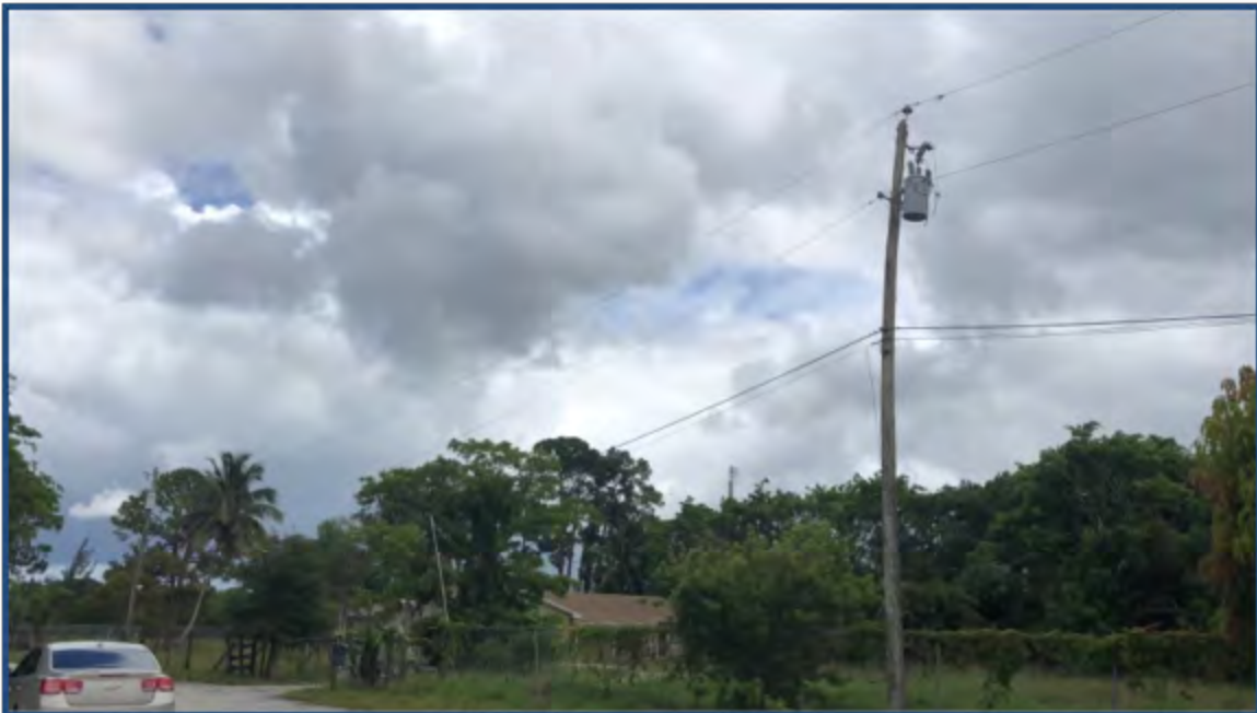
Photograph 44: Pole Mounted Transformer along 52nd court
