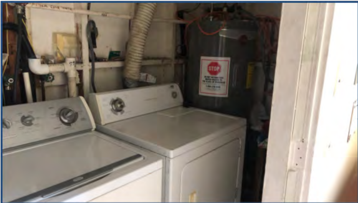
Photograph 24: Washer and Dryer Unit; and Water Heater
