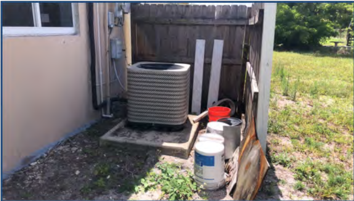
Photograph 10: HVAC System and Empty 5-Gallon Containers on North Side of Single-Family Home
