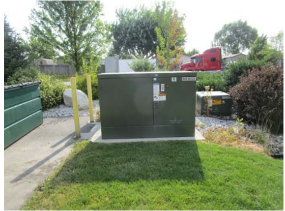
Photo #16 View of pad mounted transformer located on the southwest corner of the site.
