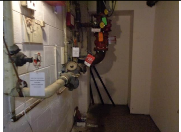
(16) View of Sprinkler Room
