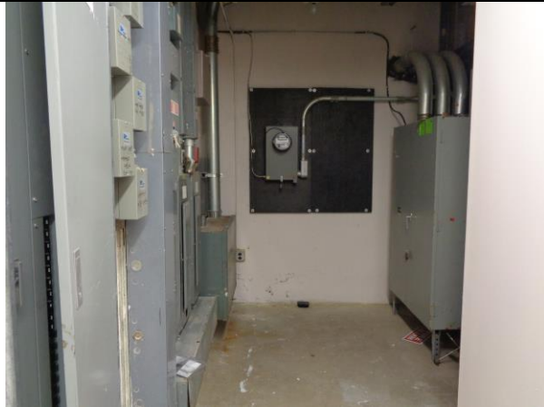
(15) View of Electric Room
