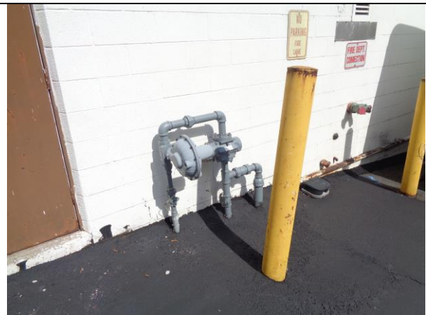
(24) View of Gas Meter
