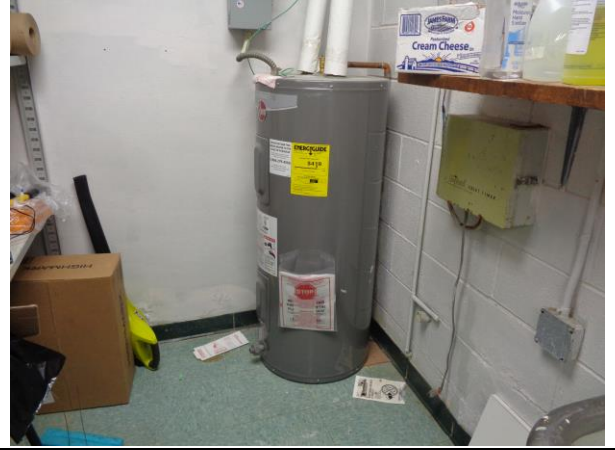
(14) View of Water Heater
