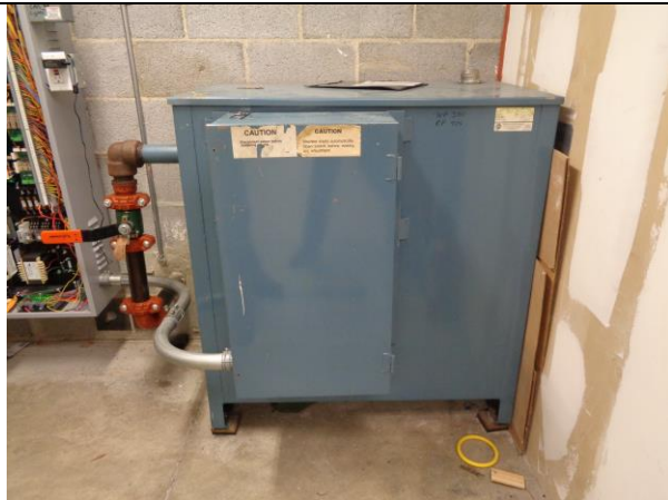
(17) View of Hydraulic Elevator Machine
