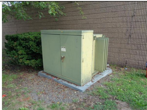
(23) View of Pad-Mounted Transformer
