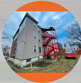
Solid Steel Fire Escape
