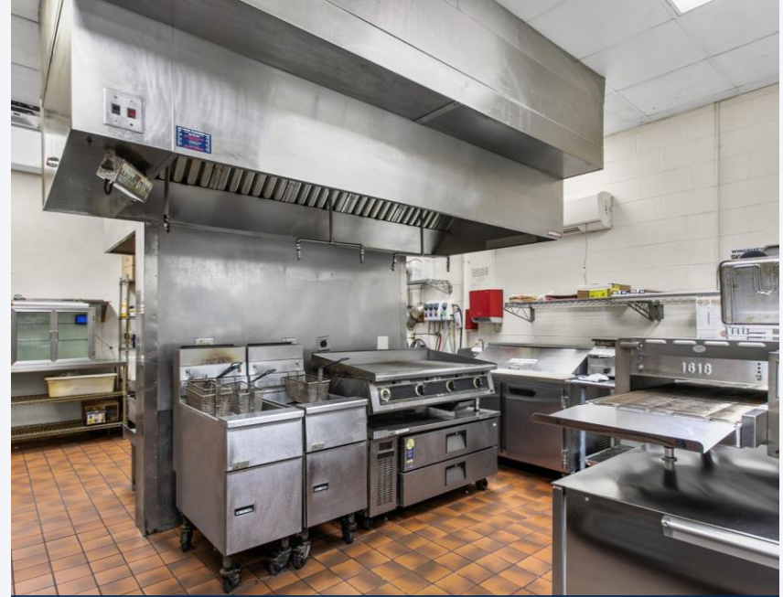
Fryer & Griddle Cook Line
