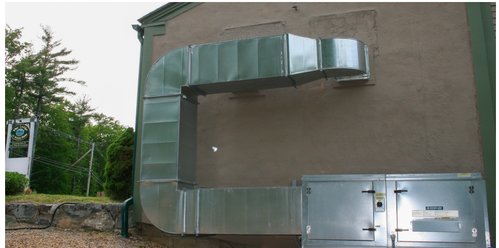
Heat & Return air for the hood vent
