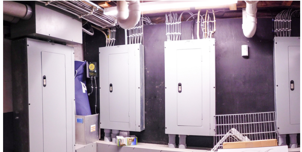
Three Phase power, electric upgraded
