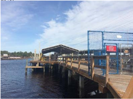
View of Cafeteria Parcel Dock over Submerged Land (Photo Taken on November 1, 2018)
