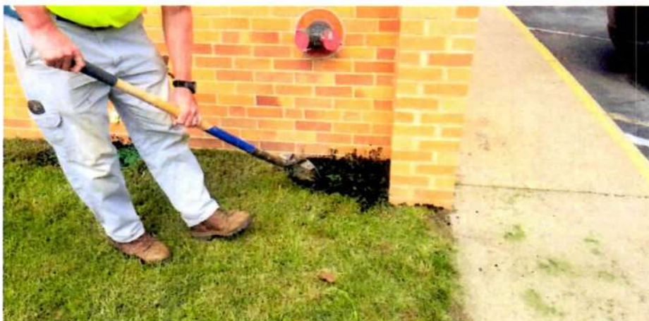
View of vent pipe, reclaimed. Taken from south, facing northeast, on 9/20/2018.
