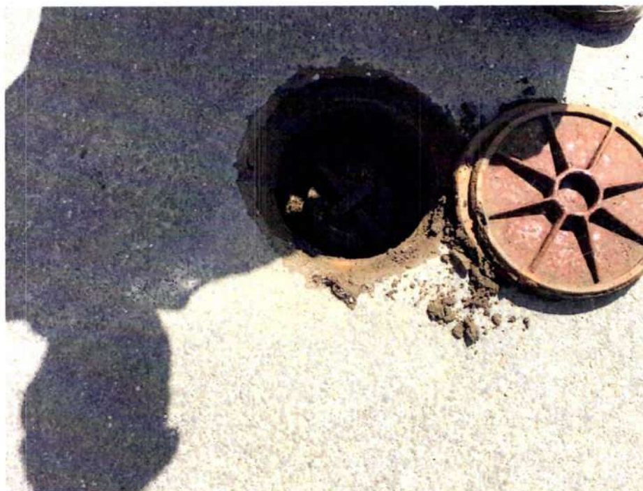
View of the 1,000-gallon UST fill pipe. Photo taken on 8/14/2018.
