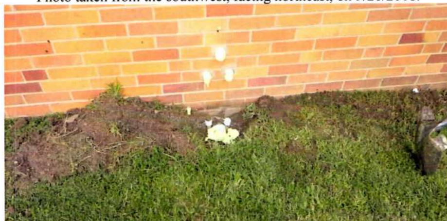
View of the product piping lines, sealed. Photo taken from the southwest, facing northeast, on 9/20/2018.
