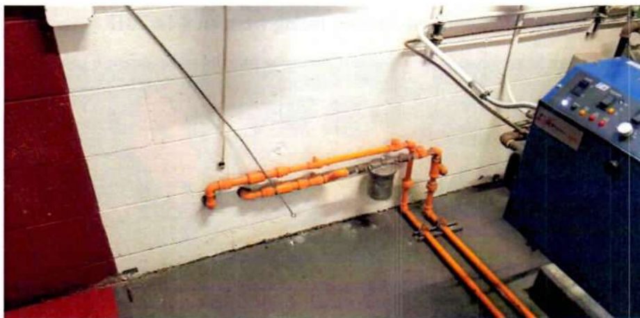
View of indoor #2 fuel oil piping to the furnace. Photo taken from the north, facing south, on 8/14/2018.
