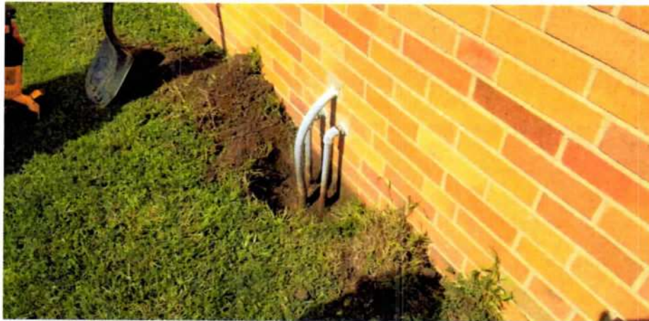
View of the product piping lines leading into the building. Photo taken from the southwest, facing northeast, on 9/20/2018.
