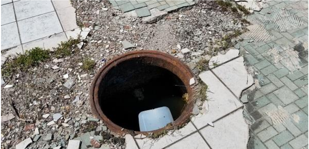
Photo 9: Open drain on property
