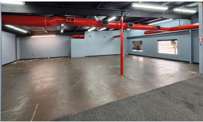
North space showroom
