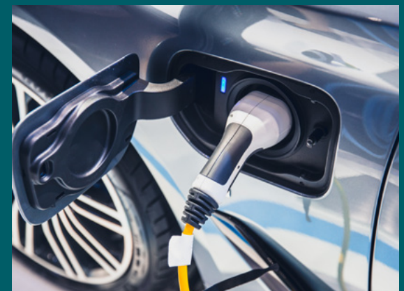
FLEXIBLE PARKING WITH 5 EV CHARGING STATIONS
