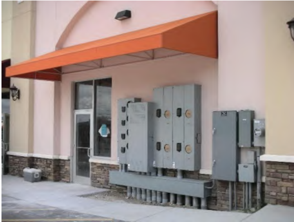
Not Allowed (utilities facing street)
