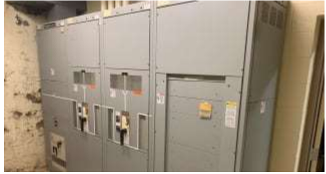
MAIN ELECTRIC PANEL
