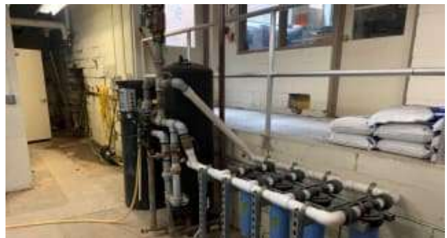
WATER SOFTENER SYSTEM
