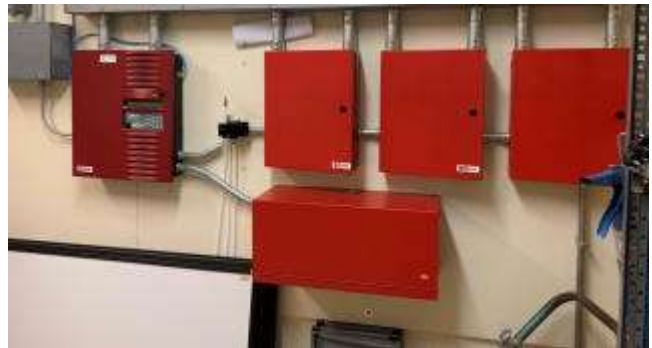
FIRE ALARM SYSTEM
