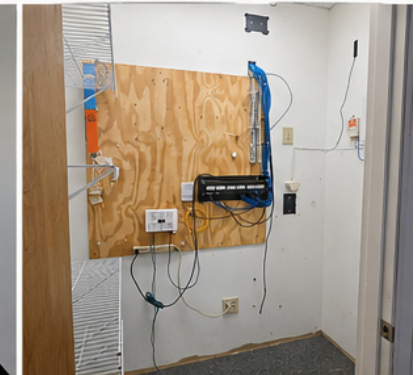
DEDICATED TELECOM / IT CLOSET
