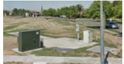
Storm pump station
