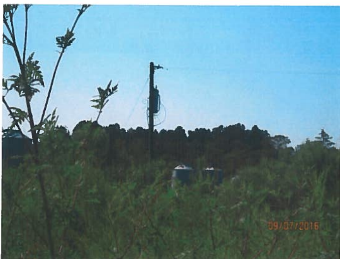
Pole mounted transformer near former chicken houses
