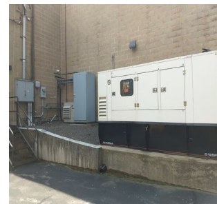
125 KVA diesel Generator
