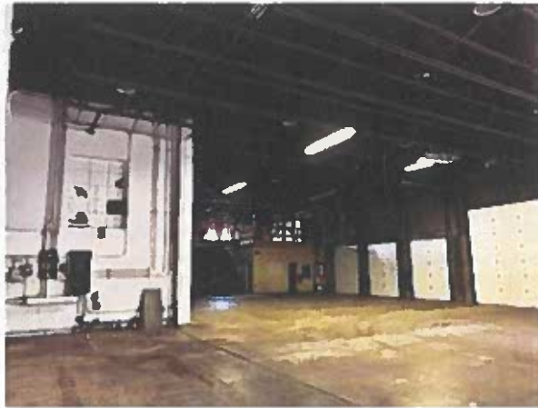
Other - View of electrical panels.
