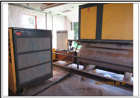
Air Compressor building interior
