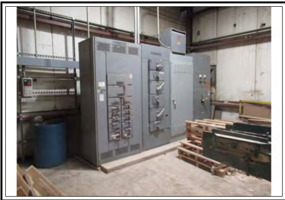
Main electrical entrance
