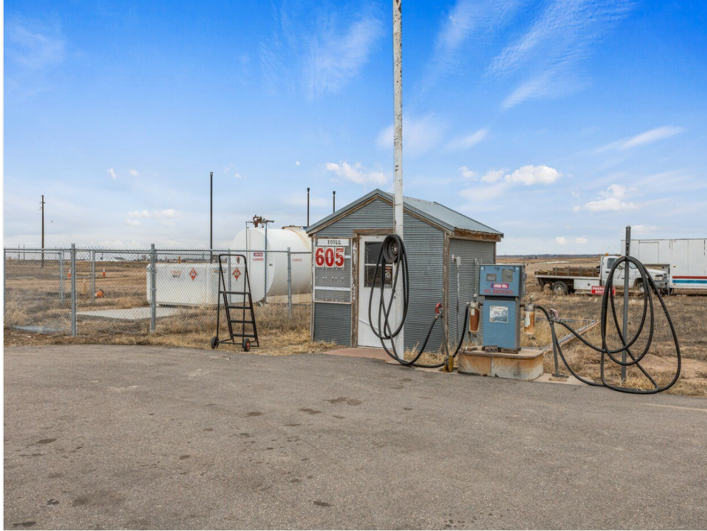
Privately Owned Self Service Fuel System
