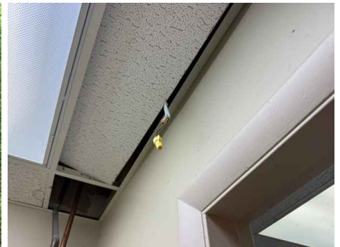
Small Utility Room
