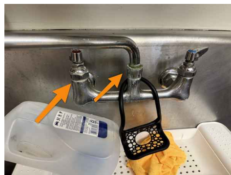
Leak at Hot Water
