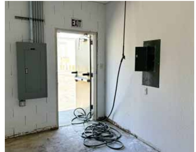
1156 N. Capitol Avenue - NEW 200 Amp Electrical Panel
