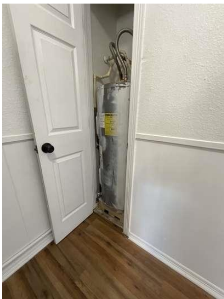
Hot Water Heater
