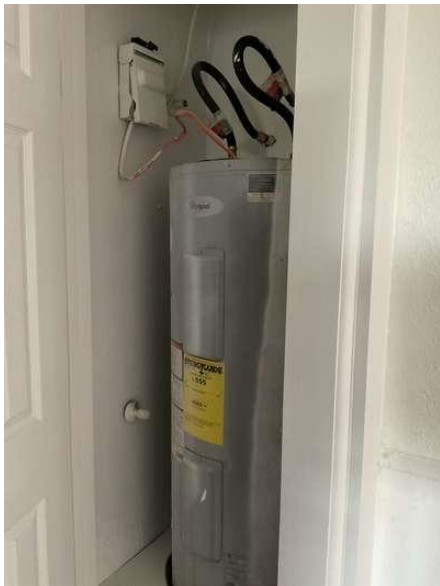
Hot Water Heater
