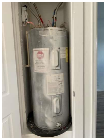
Hot Water Heater in Each Unit
