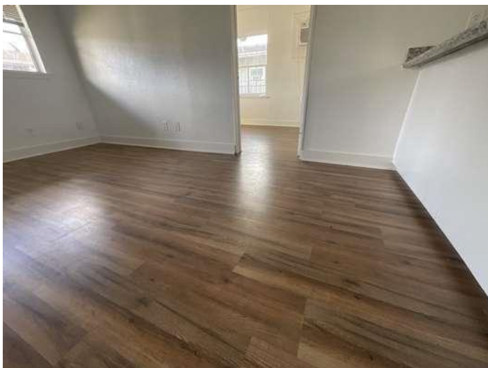
Floor slightly sloping in upper unit of West Bldg reflecting possible settlement
