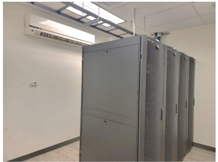
IT server room with split AC system
