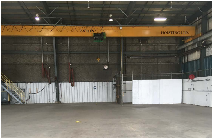
3 x 7.5 T Cranes Full Shop Coverage
