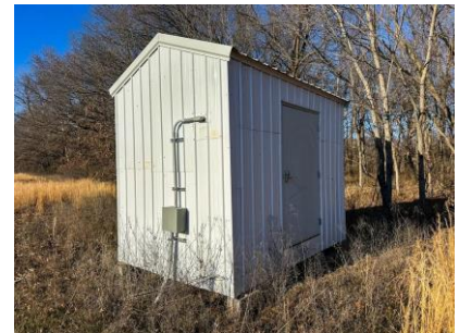
Geothermal HVAC system, 450 GPM river water available
