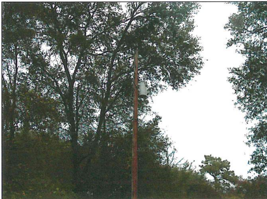
6. View of Transformer and Power lines running Through Property.
