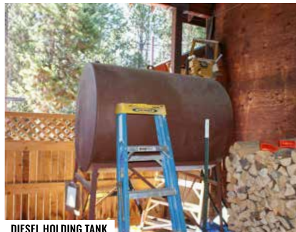
DIESEL HOLDING TANK
