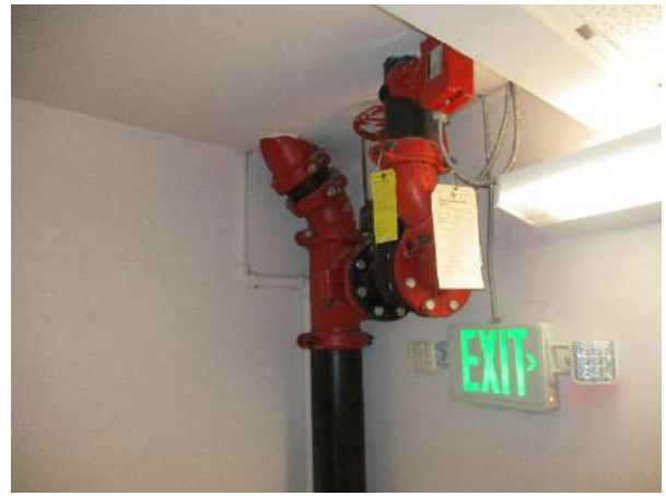
Sprinkler System in Stairs
