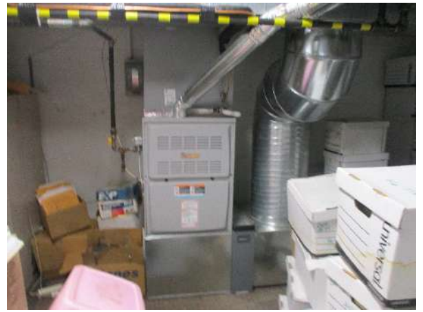
Furnace in Basement
