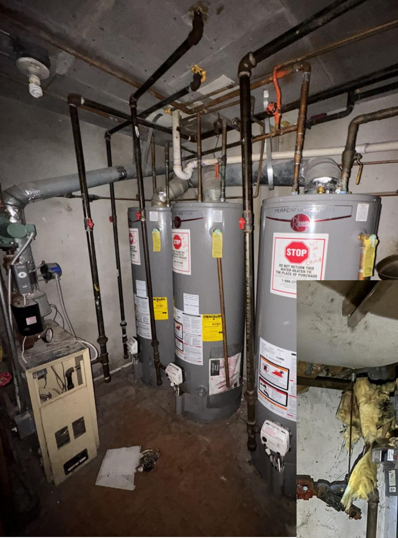
3 HOT WATER TANKS
