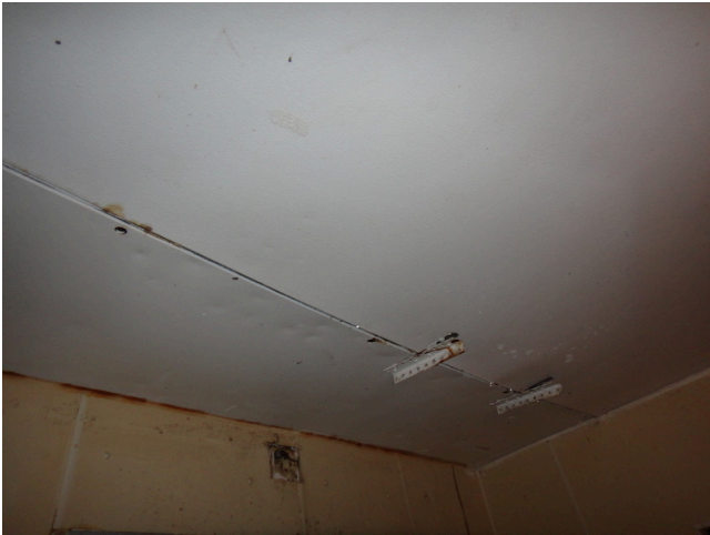
15. Roof leak bldg 1
