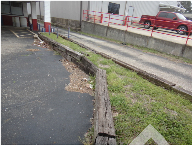
9. Damaged wood landscaping borders
