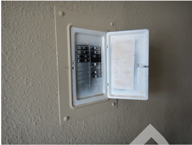
25. Circuit breaker panel
