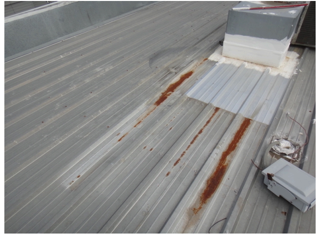
14. Roof surface rust bldg 1
