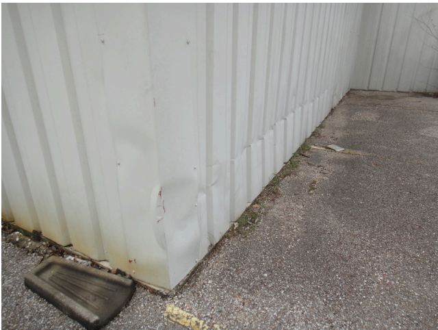
43. Metal panel wall damages
