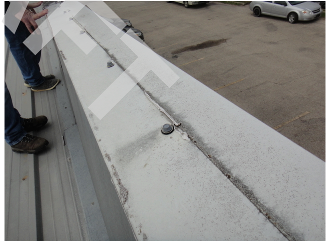
16. Roof coping poor
