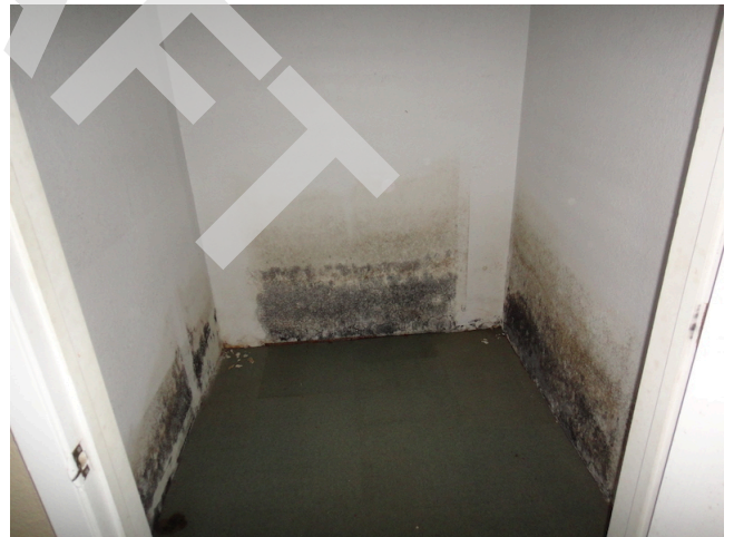
4. Mold damage bldg 2
