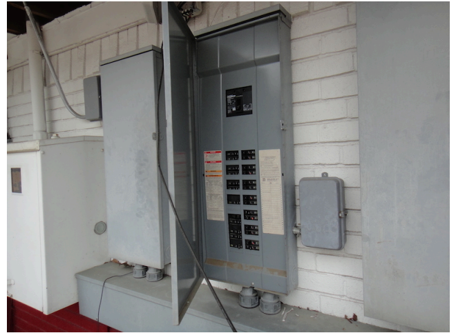
26. Circuit breaker panels bldg 1
