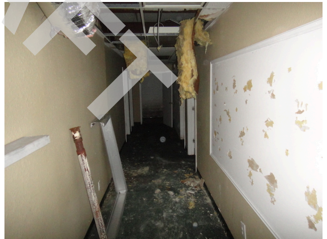
20. Bldg 2 interior poor
