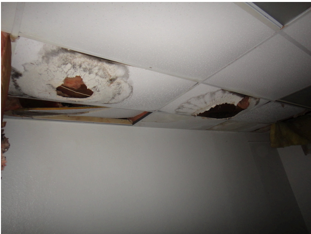
19. Past roof leaks bldg2
