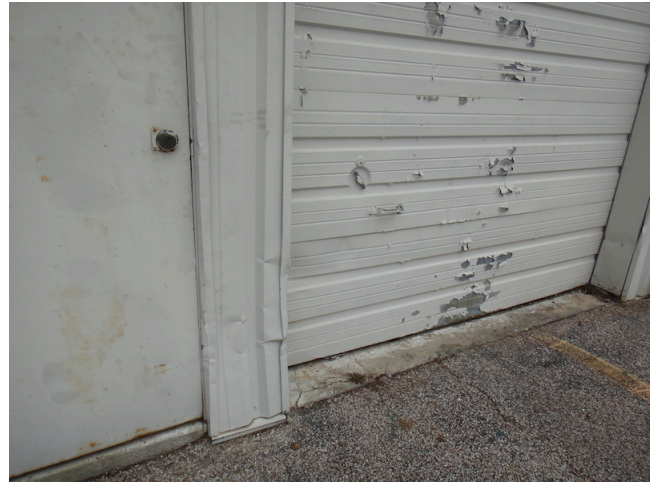
10. Fair to poor finishes
