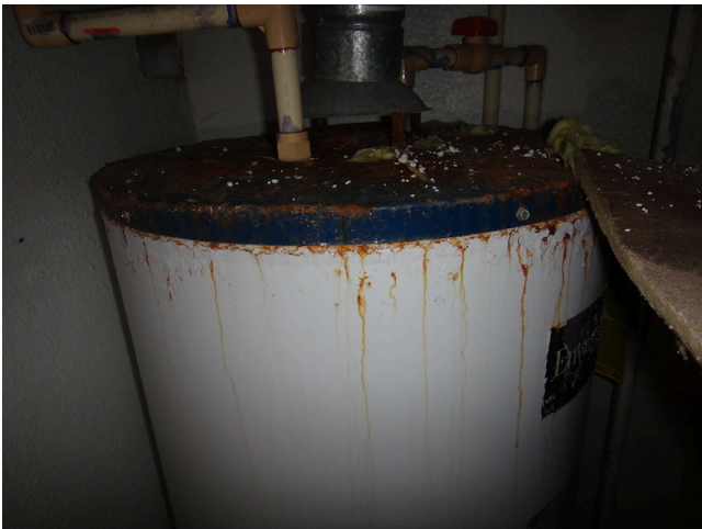
47. Poor water heater
