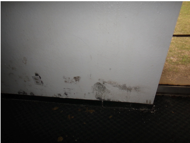
3. Moisture damage bldg 2
