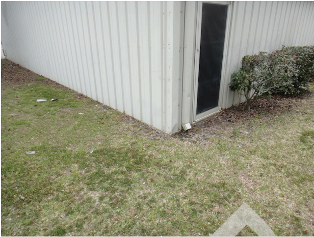
5. Poor drainage along southeast
