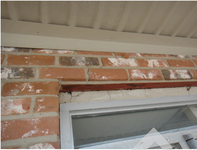
61. Minor brick crack at bldg 1
