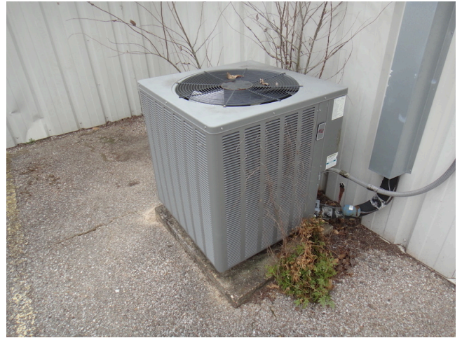
54. Split system HVAC
