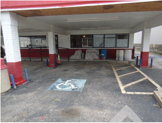
21. ADA signage needed
