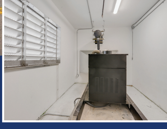
Full-Building Natural Gas Generator
