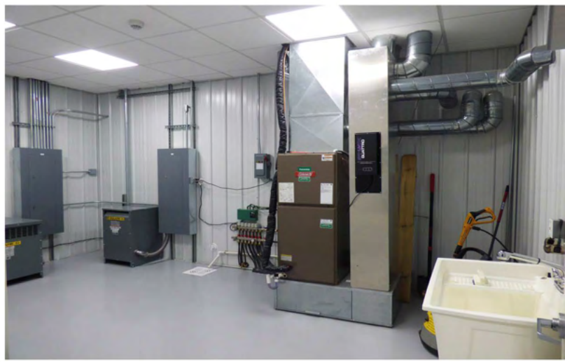
EAST MECHANICAL ROOM
