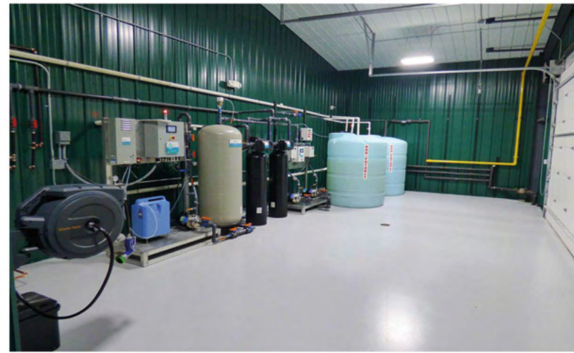
OZONE WATER TREATMENT PLANT
