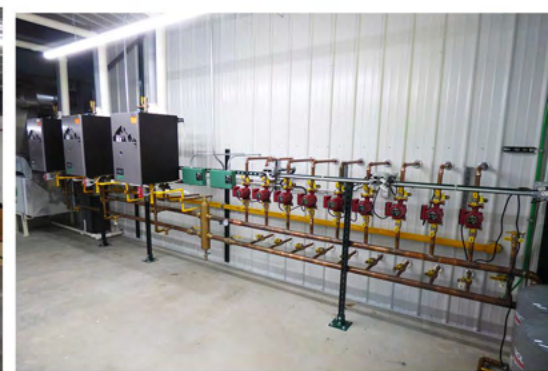
IN FLOOR RADIANT HEAT
