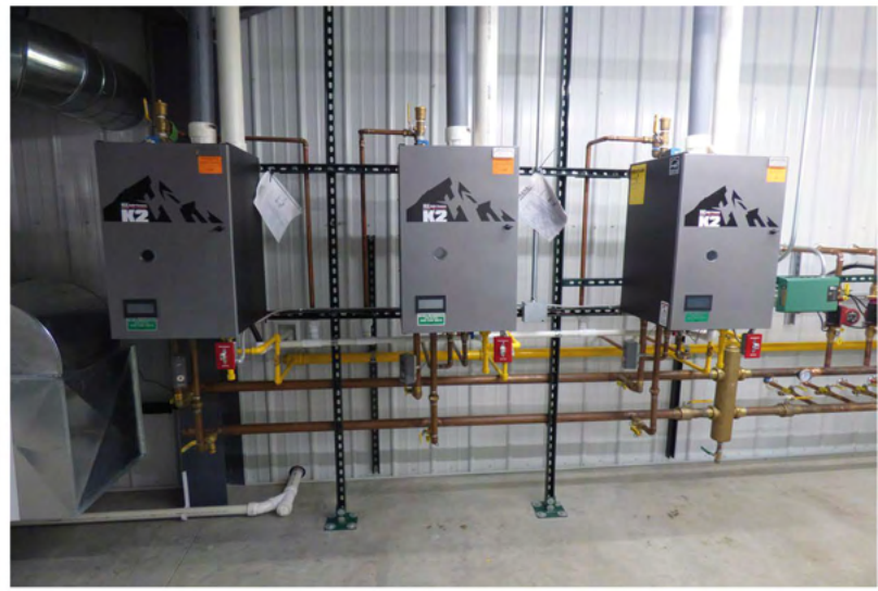
BURNHAM K2 BOILERS
