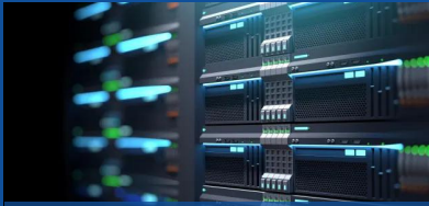
Integrated Tech and Server Room
