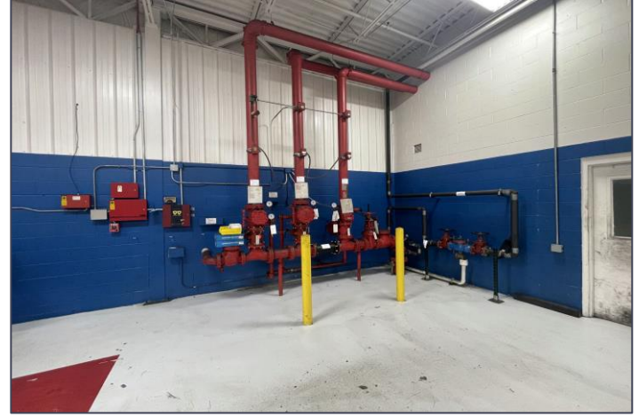
Fire Suppression System
