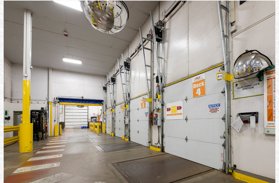
4 RECESSED LOADING DOCKS WITH SERCO MASTER CONTROL PANELS
