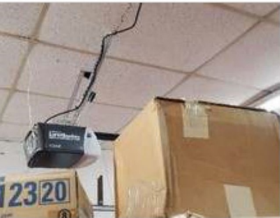
Rear side overhead door opener
