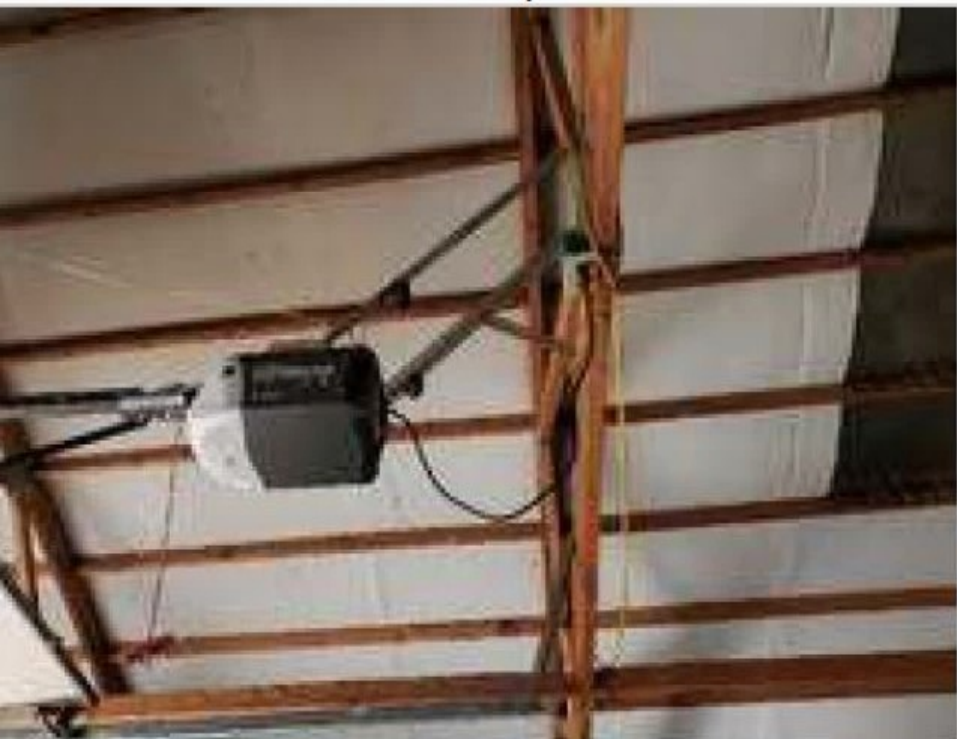
Large building overhead door opener
