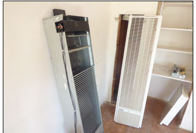
Unit 430 – Wall Heater
