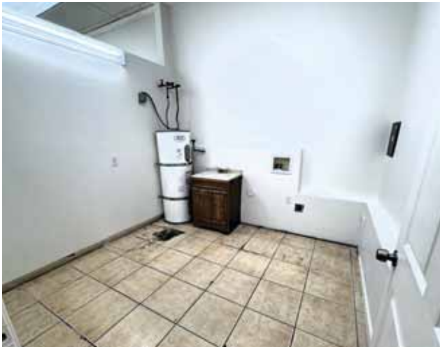
Dispensary Rm 50-Gal Hot Water Heater / Washer Hookups
