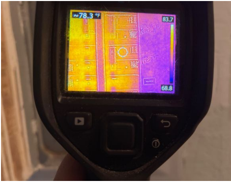
General Info: Main Breaker / Service Disconnect Location At Main Breaker by Exterior Meter
