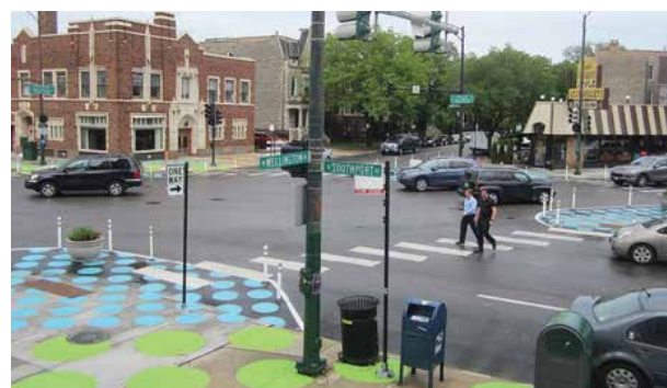
Public art can be integrated into curb extensions. (Source: John Greenfield; from Quick Builds for Better Streets, PeopleforBikes)
