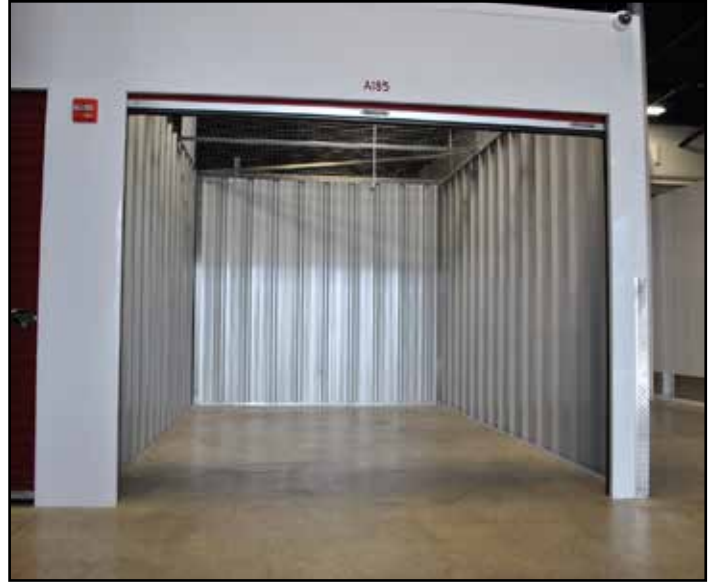
6a. 29 gauge vertical galvalume partition located inside units. (Center girt not required.)
