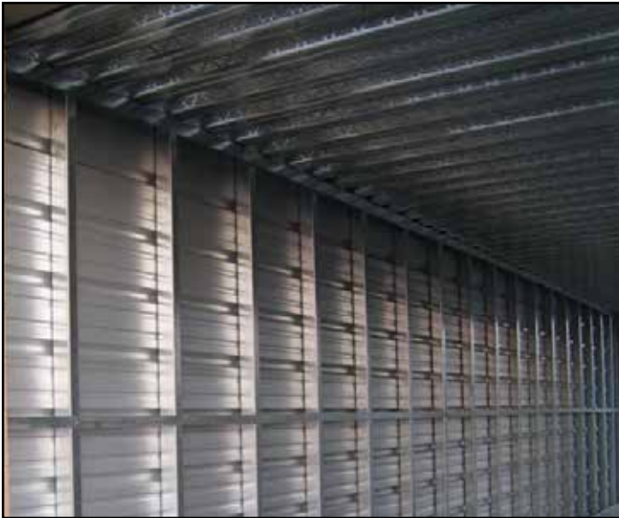
11b. Multi-floor galvanized stud wall structure includes horizontal galvalume partition panel to under side of floor deck. The partition may be held down (normally 18") to allow for sprinkler system. This option has an additional cost.
