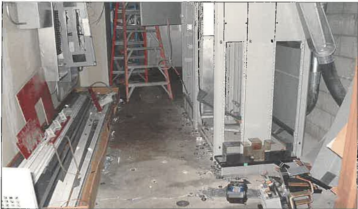
VANDALISM IN THE ELECTRIC ROOM
